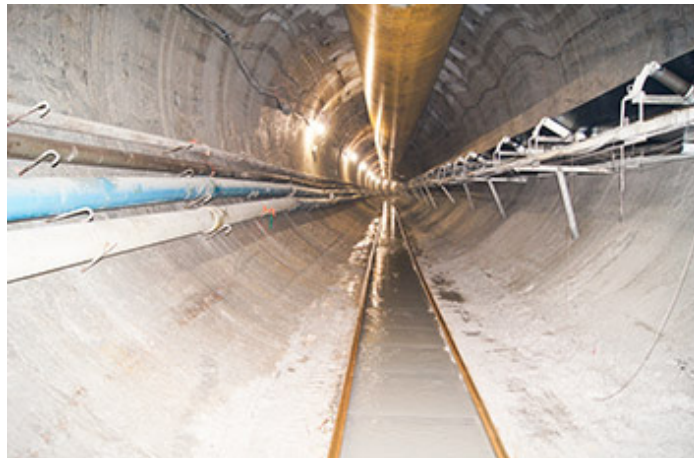
Standardizing the width of tunnels at 20 feet, 2 inches reduced the cost of the DigIndy project about $50 million. (Photo courtesy of Citizens Energy Group)
